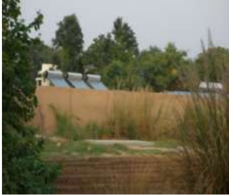
Solar water heater combined with water treatment to save energy and water
