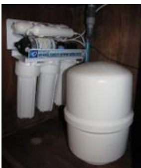
Reverse osmosis provides drinking water in every guest room.
