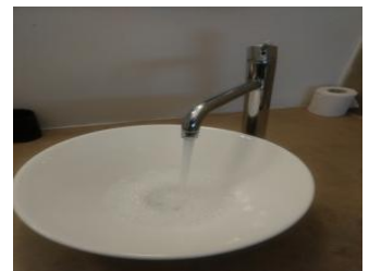
Aerated taps, one of several measures to conserve water.
