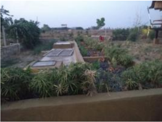
Phytorid water treatment...
