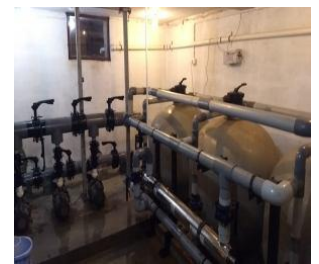
UV filter is used to treat water from the swimming
