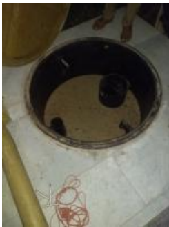
Grease trap behind the kitchen.
