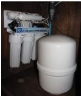
Reverse osmosis provides drinking water in every guest room.
