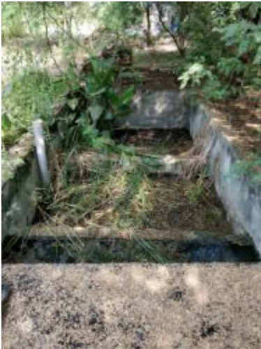
Phytoremediation wastewater treatment.
