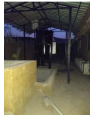
ETP Unit for laundry wastewater.
