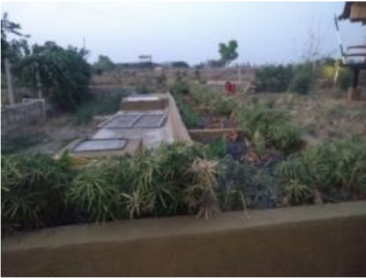
Phytorid water treatment...
