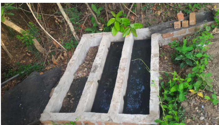
Gravel, sand and charcoal filtration pit to clean grey water from washing and overflow pits before releasing into nallah sand beds.
