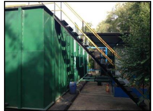
STP at Oberoi Vanyavillas. See case study.
