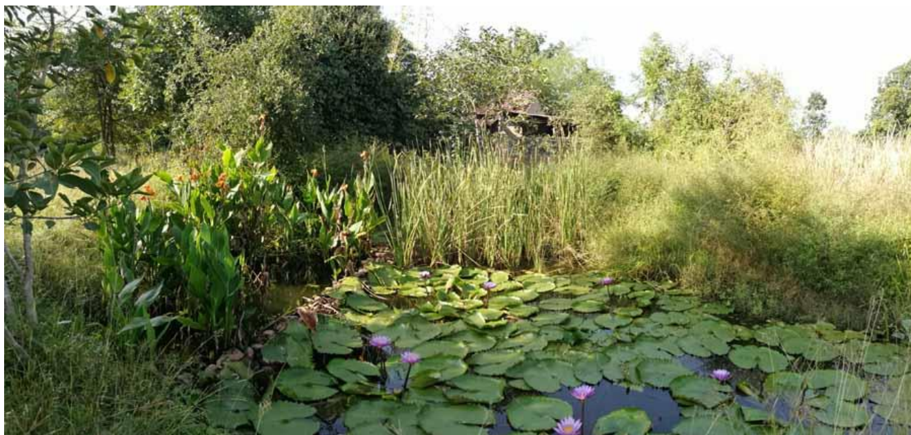
Reed bed system to filter grey water from the kitchen.
