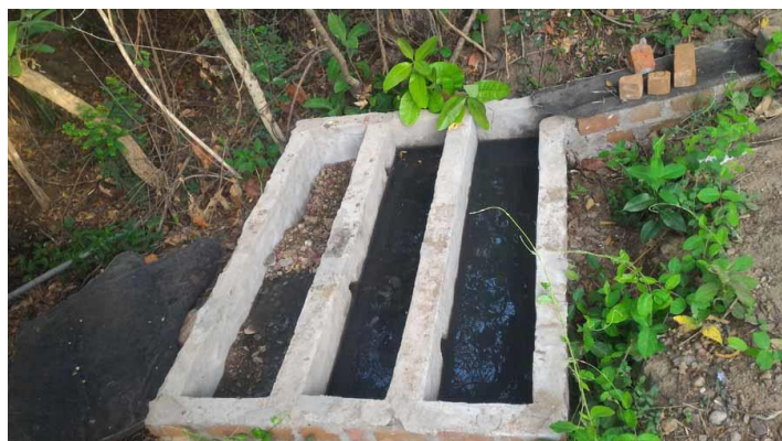
Gravel, sand and charcoal filtration pit to clean grey water from washing and overflow pits before releasing into nallah sand beds.
